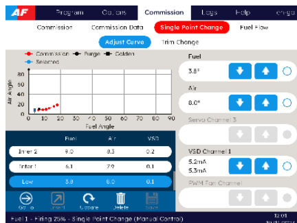
Single point change for commissioning
